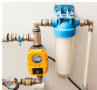
Funds are now available for automatic water shutoff and leak detection systems.
